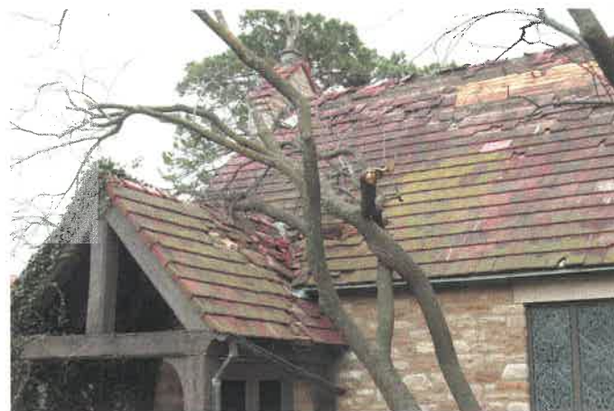
Danforth Chapel sustained major roof damage – Mike Krings, Doug Koch/University Relations
