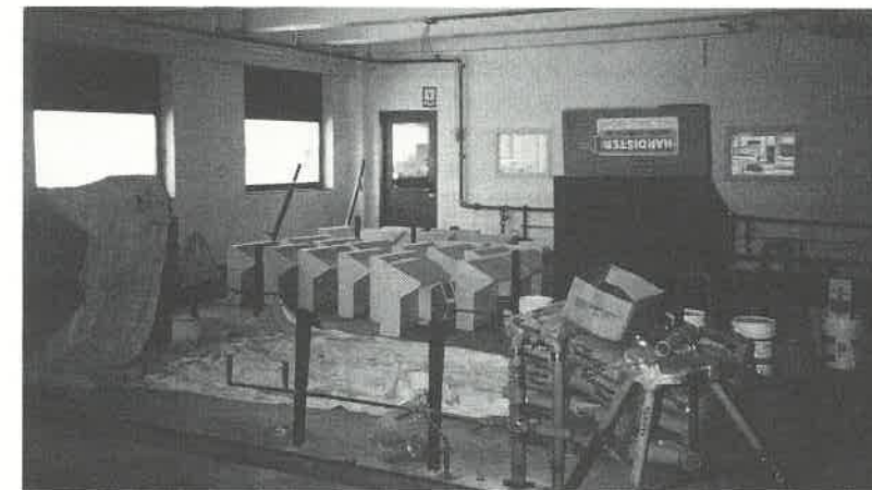
This is the final summer for crumbling classroom repairs. The third floor CHEM 517 Analytical Chemistry laboratory is one of several being remodeled this year. Behind the small windows in the rear wall is the Department's new Instructional Instrumentation Laboratory.
