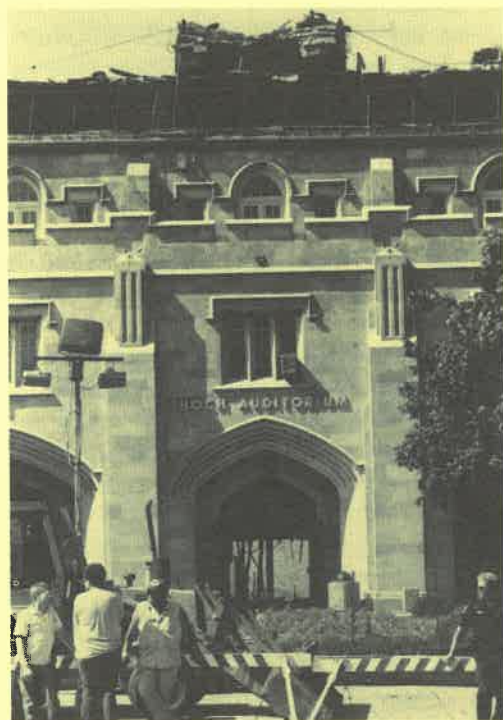
View of the main entrance to Hoch a few days after the fire. The appearance is still much the same at the time of this writing. [Photo by Tim Miller]
