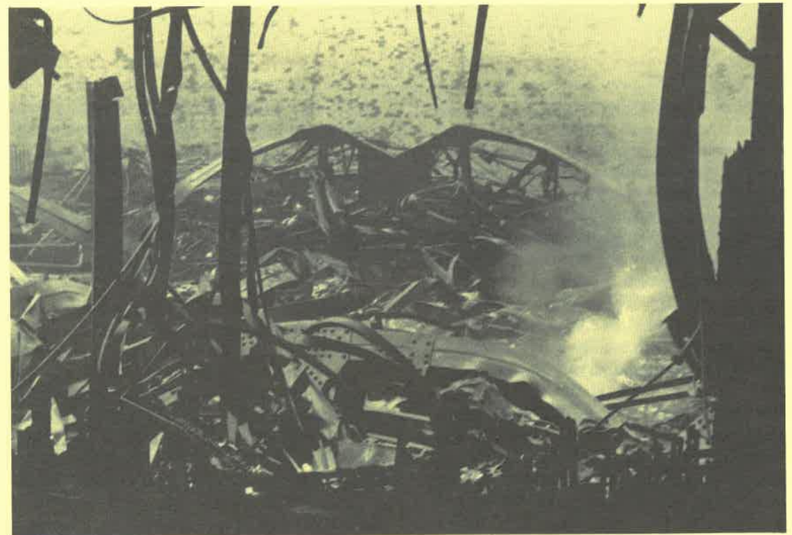
View of the interior of Hoch Auditorium after the fire. The steel beams shown once supported the roof. [Photo by Tim Miller]
